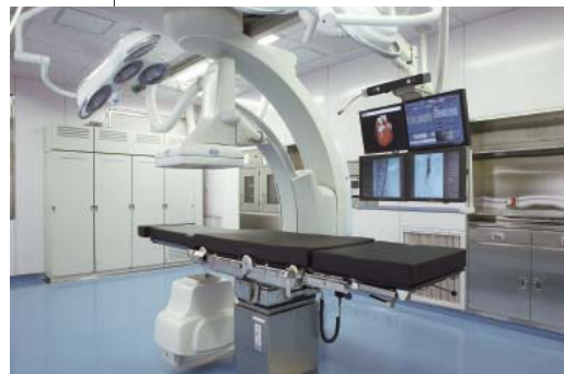
Figure 1. Hybrid operating room A radiolucent operating table (ALPHAMAQUET 1150, MAQUET) and a ceiling mounted C-arm with FPD (TOSHIBA Infinix™-i INFX-8000H Angiographic imaging system) are installed in the hybrid operating room. This room can also be used for cardiovascular X-ray diagnosis and interventional procedures.
